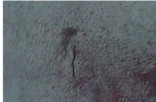
Fig. 9.19: A crack indication detected after inspection.
