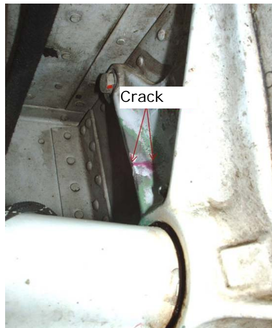
Fig. 8.8: A crack indication that appears after the test.
