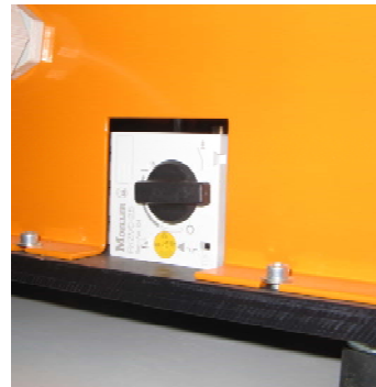
Fig. 5.7: The machine ON/OFF switch.
